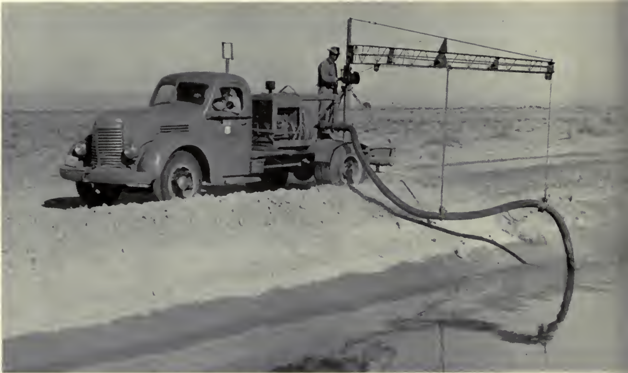
LONG DISTANCE ROAD SPRINKLING is much more efficient with this type of equipment. Photo by Maurice N. Longley, Region
